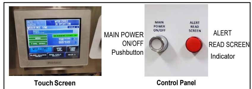
Figure 5-2. Pro Cleaning System Controls (Typical)
