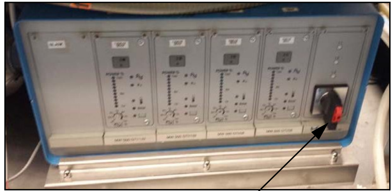
Generator Power Switch
