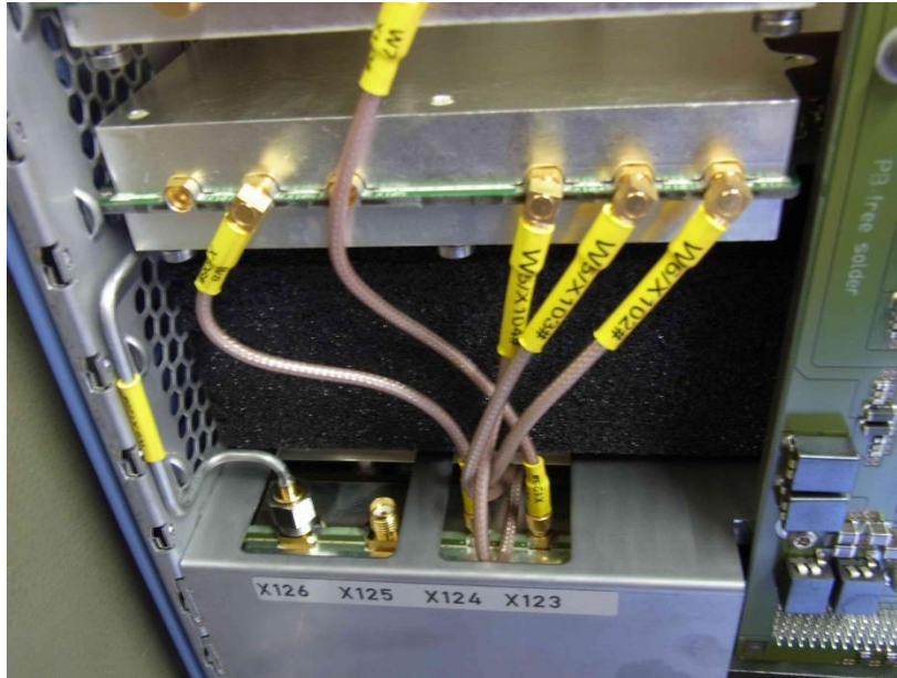
Figure 4-18: Cable routing without option R&S®FSW-B71 and without option R&S®FSW-B1200 installed
