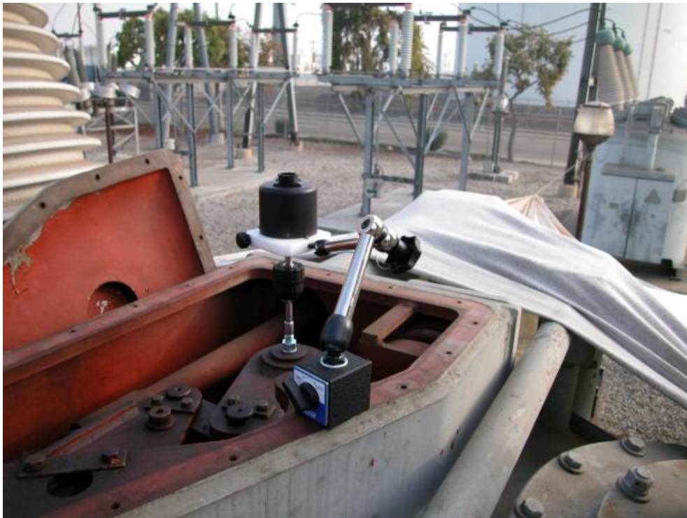
Rotary transducer on Federal Pacific Circuit Breaker
