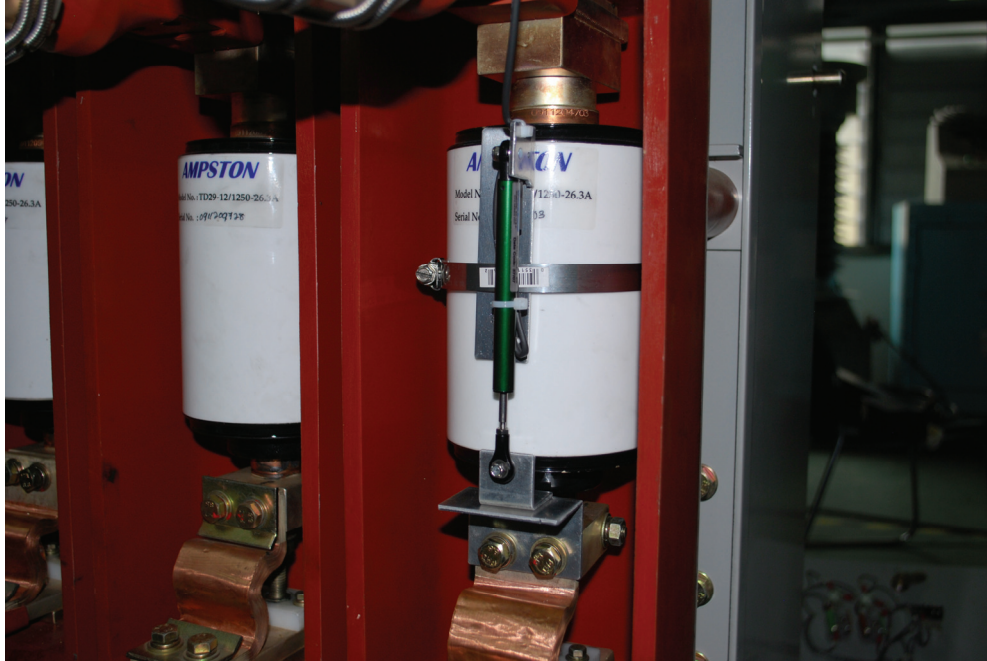
Resistor Transducer on Vacuum Circuit Breaker
