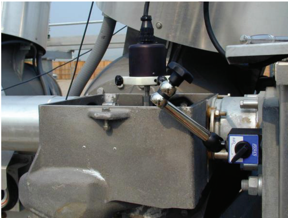
Rotary Transducer on Alstom HE 1014 Circuit Breaker
