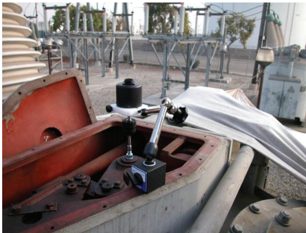
Rotary Transducer on Federal Pacific Circuit Breaker
