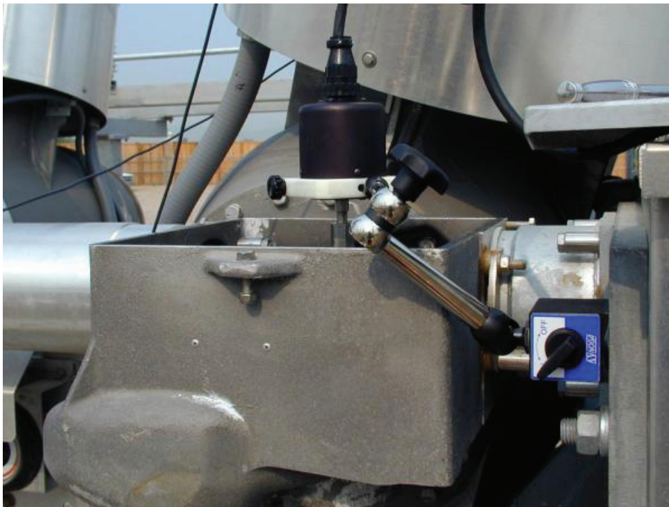
Rotary Transducer on Alstom HE 1014 Circuit Breaker
