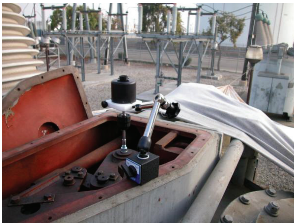
Rotary Transducer on Federal Pacific Circuit Breaker
