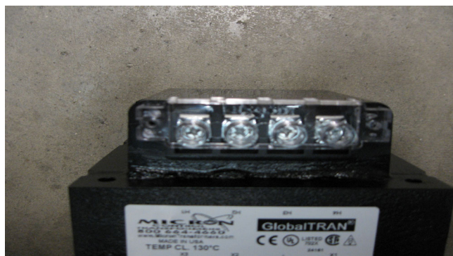
FIGURE 5.3.PRIMARY POWER WIRES TO TRANSFORMER
