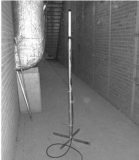
End feed antenna installed next to a kiln.
