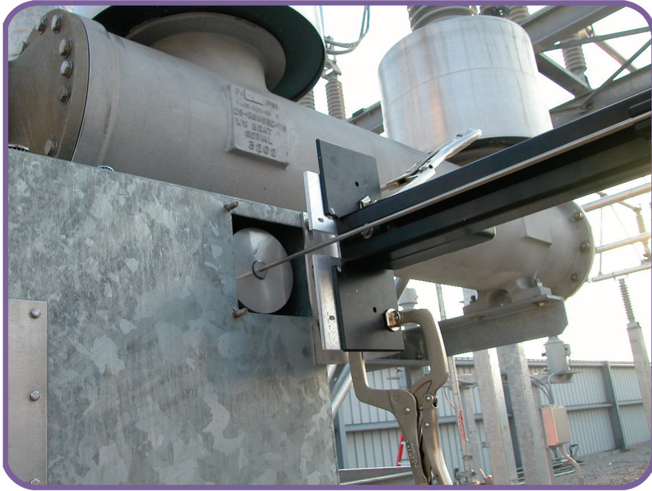
Figure 34. Linear Transducer on Areva DT1-72.5F
