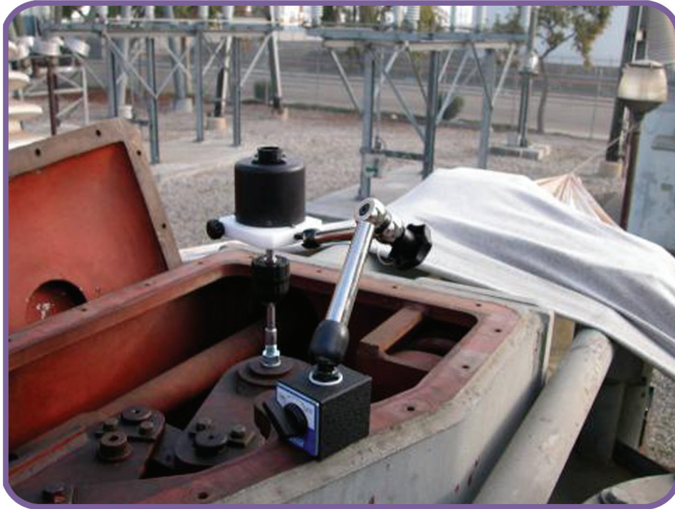
Figure 32. Rotary Transducer on Federal Pacific Breaker
