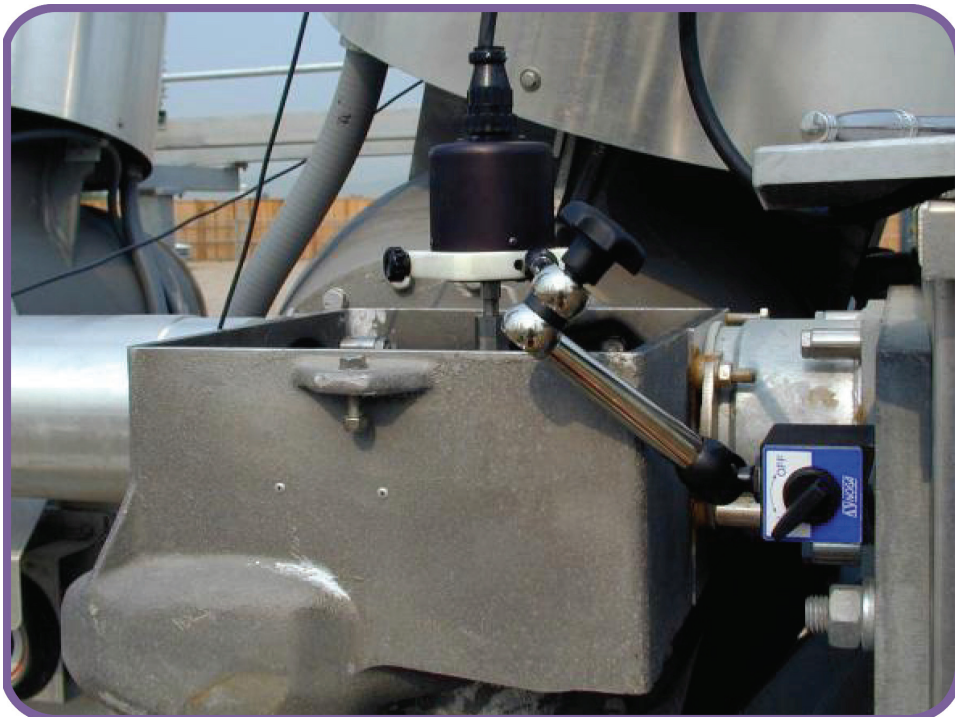
Figure 27. Rotary Transducer on Alstom HE 1014 Circuit Breaker
