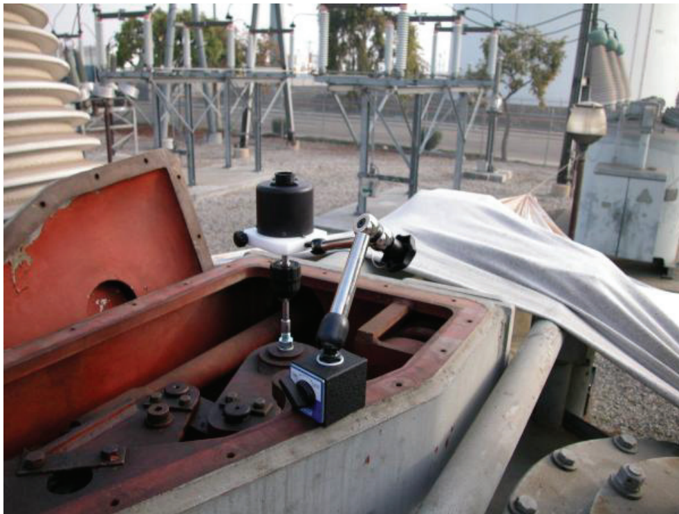
Rotary Transducer on Federal Pacific Circuit Breaker
