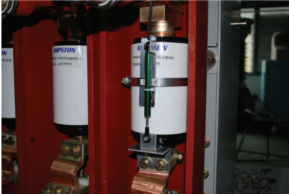
Resistor Transducer on Vacuum Circuit Breaker
