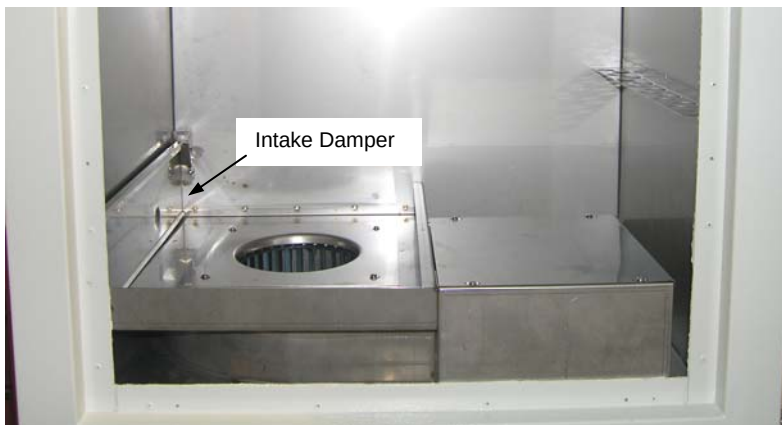
CONDITIONING PLENUM – INTAKE DAMPER FULLY CLOSED
