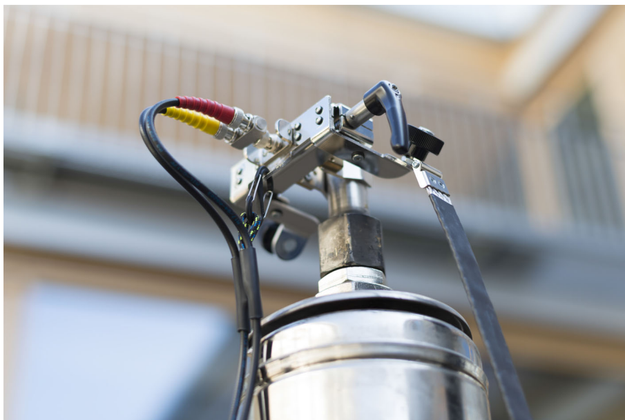
Figure 5-4: Connecting the yellow and red coaxial cables to the bushing clamp by using the mechanism for relieving the pressure on the BNC shield
