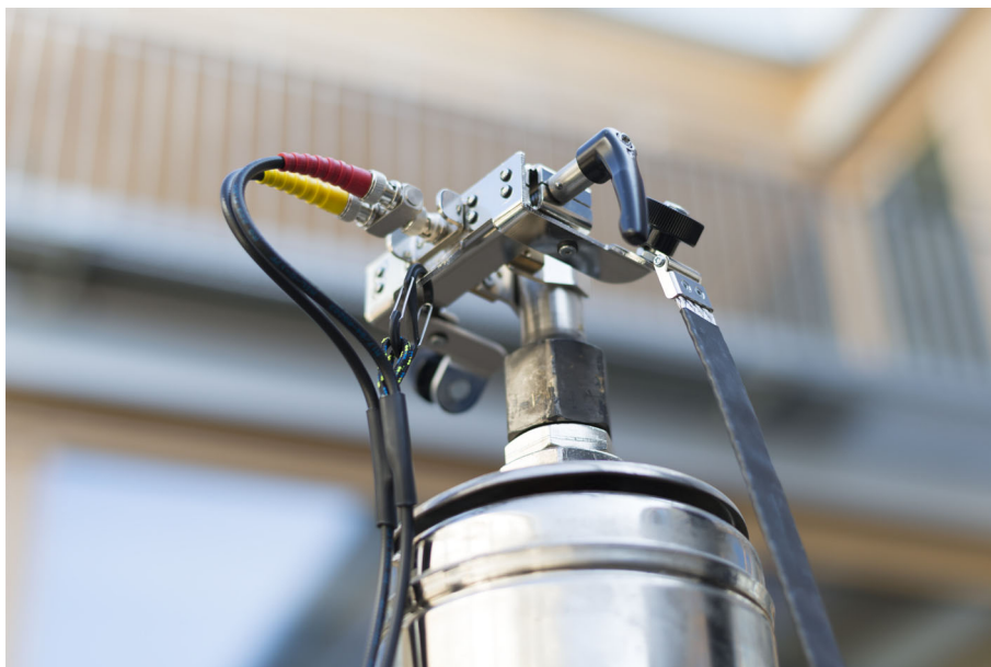
Figure 4-4: Connecting the yellow and red coaxial cables to the bushing clamp by using the mechanism for relieving the pressure on the BNC shield
