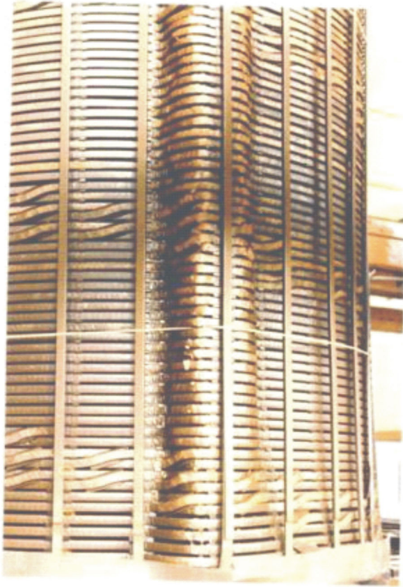
Figure 3-3: Radial coil deformation
