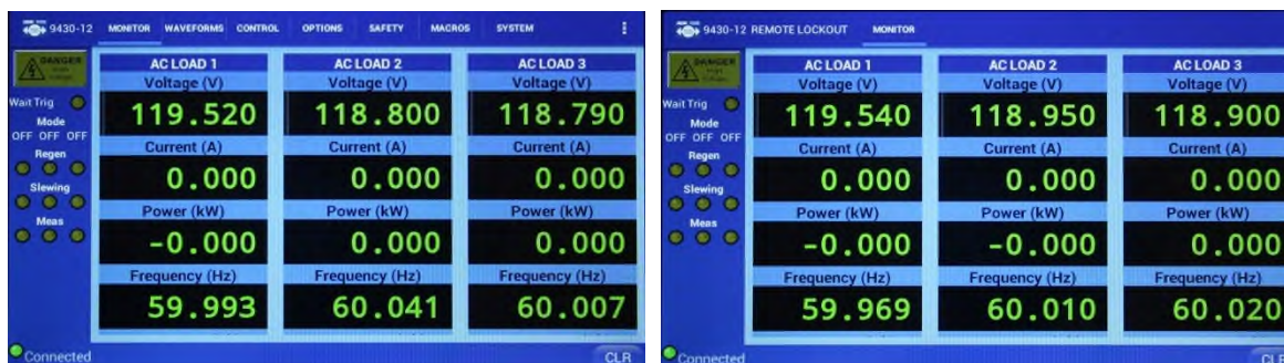
Panel is Primary Controller
