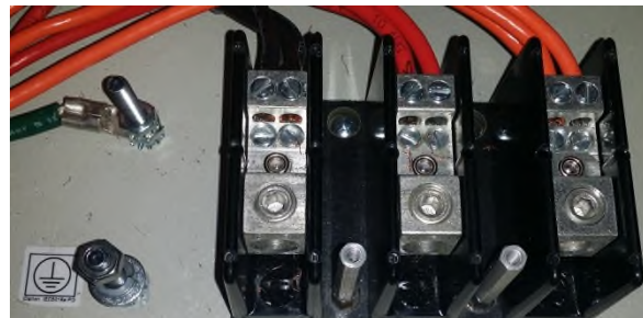
Chassis Power Connection
